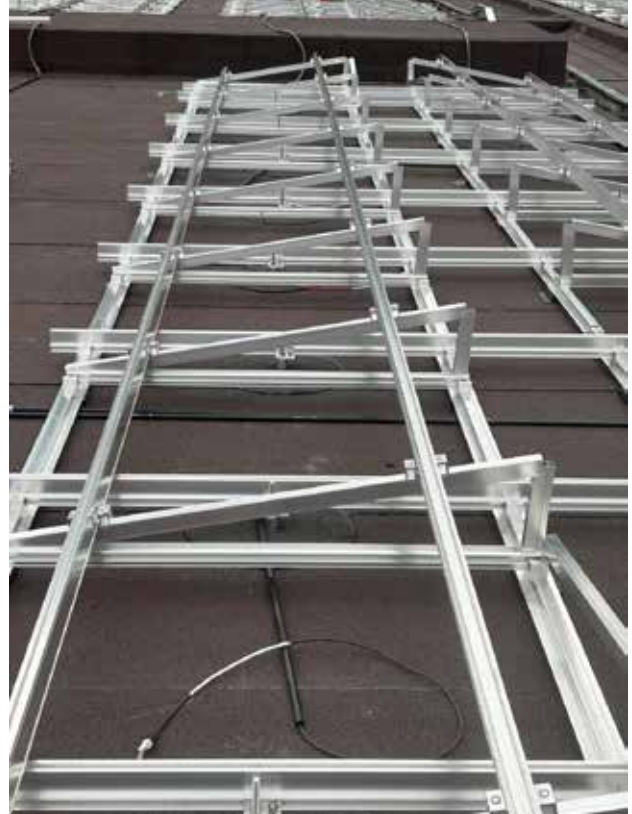
Solar Mounting Systems finalized.
