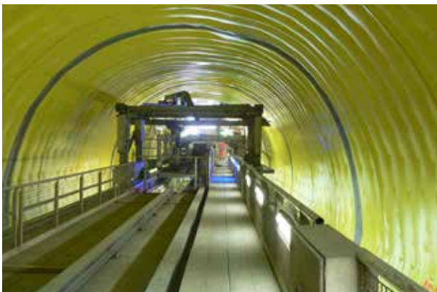
Durable waterproofing systems applied after stabilising with sprayed concrete and before the inner segment concrete lining.
