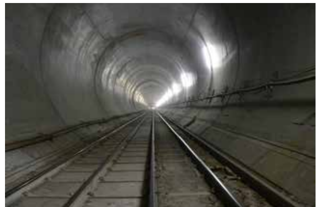
Inner segment concrete for durable final lining of the two main tubes.
