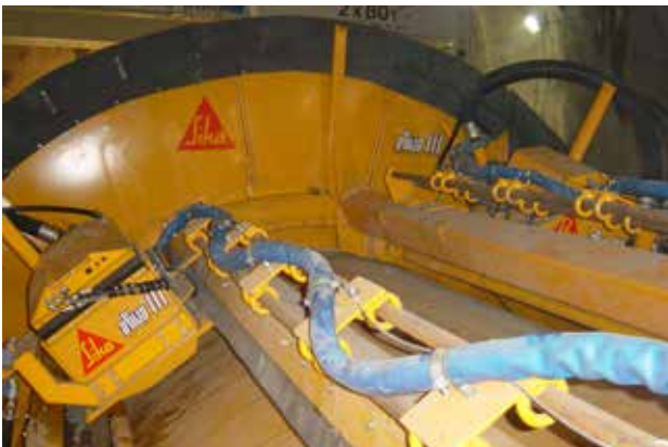
Sprayed concrete stabilisation behind the excavation with wet sprayed concrete in the TBM section.
