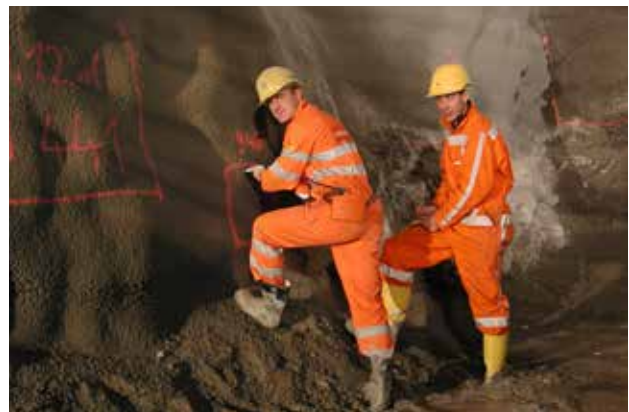
Sika specialists on site during the early strength testing of the sprayed concrete.
